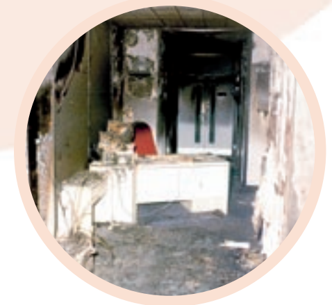
The result of an office fire
